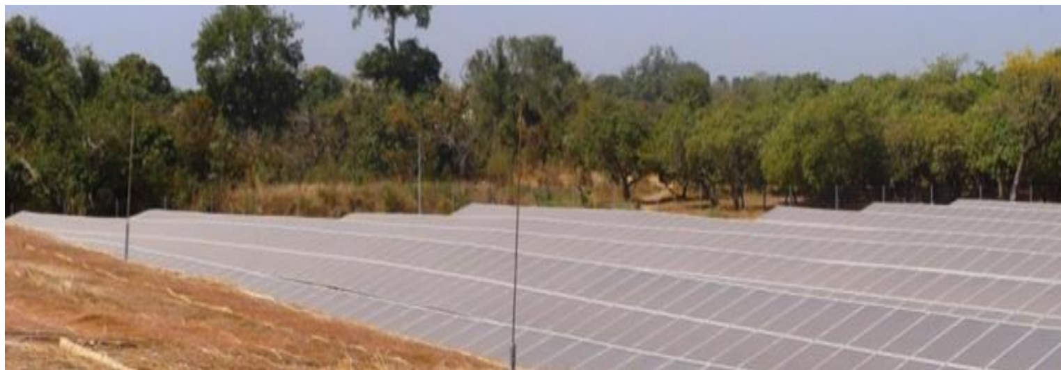
Panoramic view of the power plant
