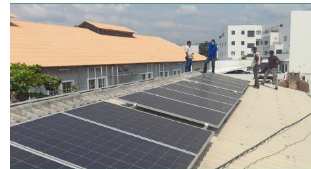
Figura 1: Painéis Solares instalados. Figure 1: Solar panel installation.
