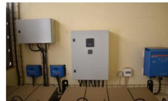
Figura 3: Painel e baterias instaladas. Figure 3: Installed system and battery bank.
