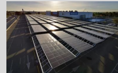
Solar PV Carport
