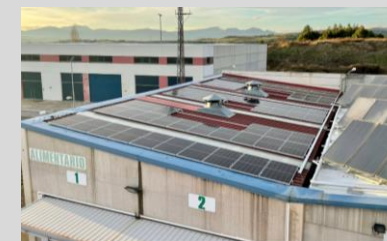
Solar PV Roof Mounted
