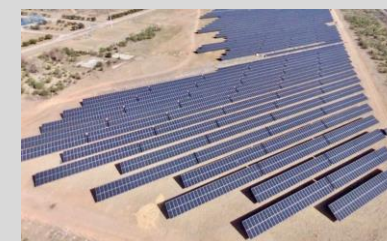
Solar PV Ground Mounted
